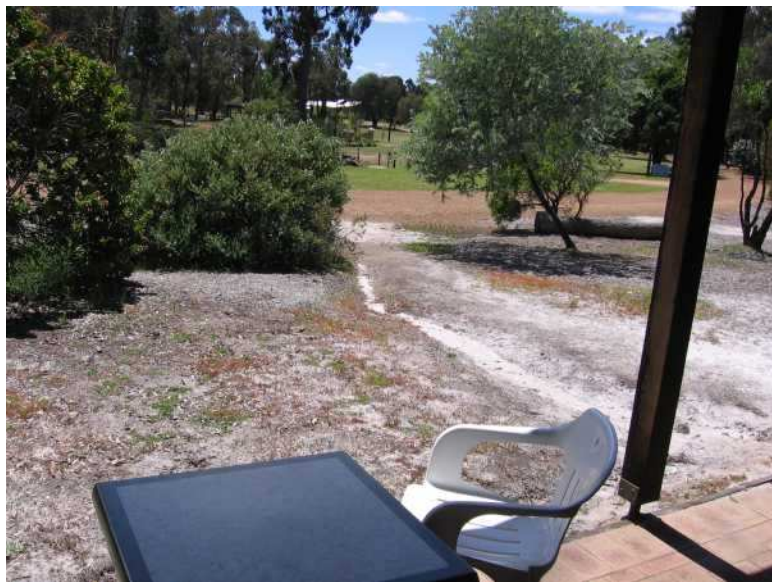
First impressions of the Park via the café entry point - sand, weeds and soil erosion.
